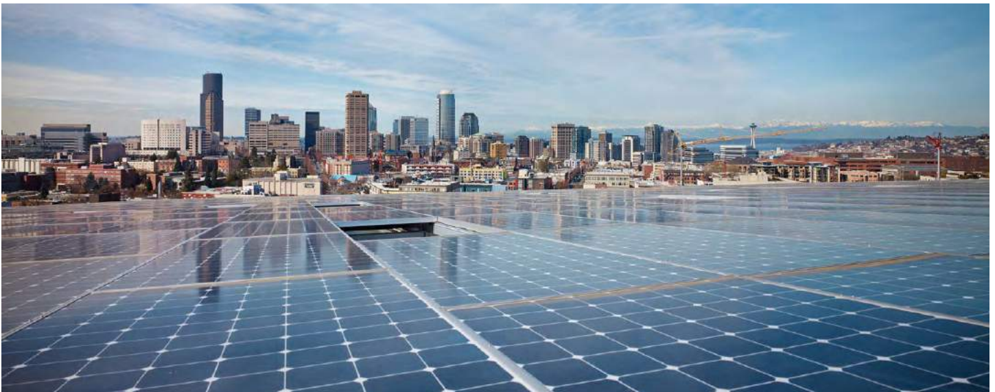
The Bullitt Center PV Array, Seattle WA
