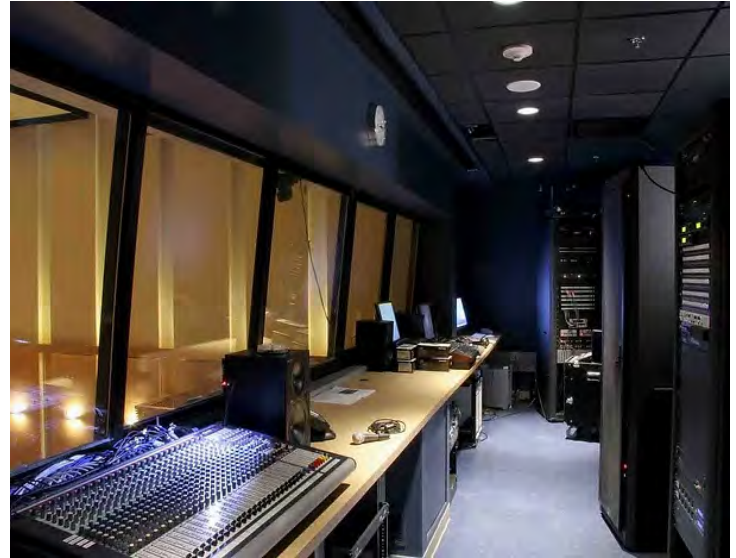
Theatre control room, Tufts University, MA - AV controls and equipment racks
