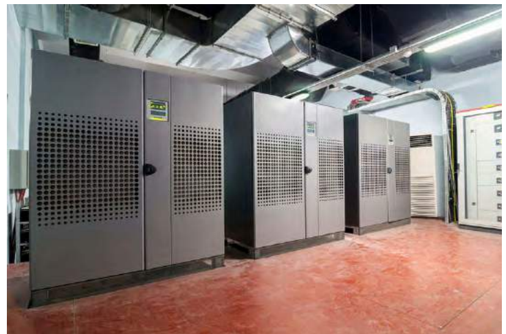
Partially finished support space with communications equipment
